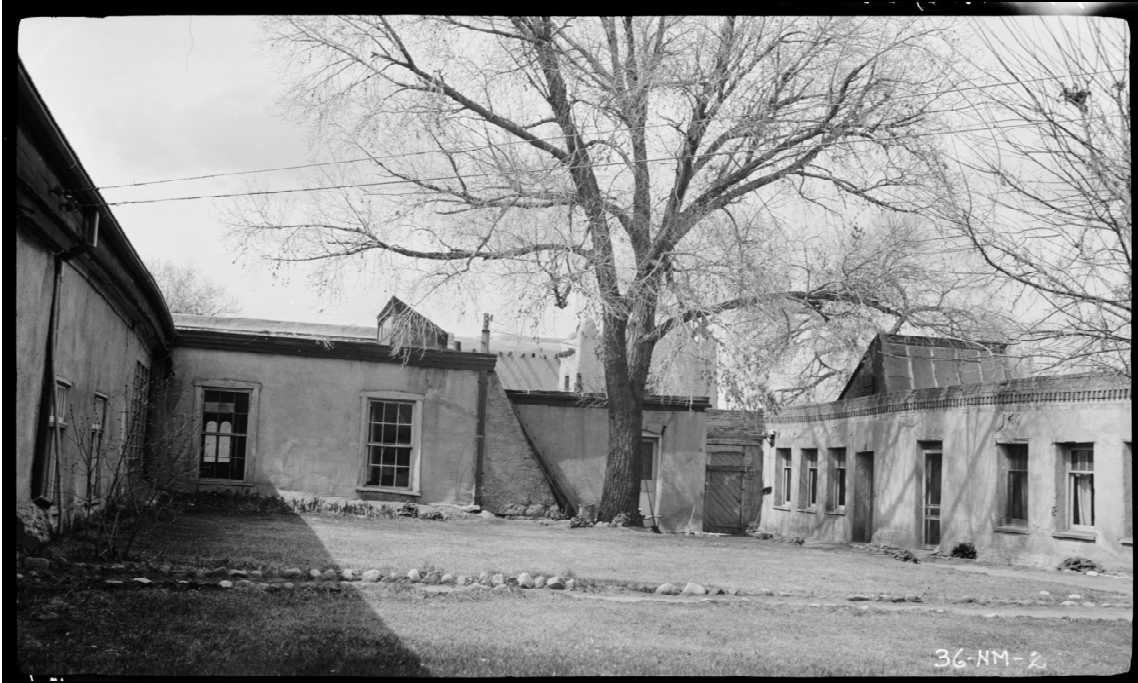
Fig. 7. Placita Looking West. Photograph by M. James Stack, 1934. Historic Building Survey. Courtesy of the Library of Congress, Prints and Photographs Division. HABS NM, 25-SanFe, 2-4.
