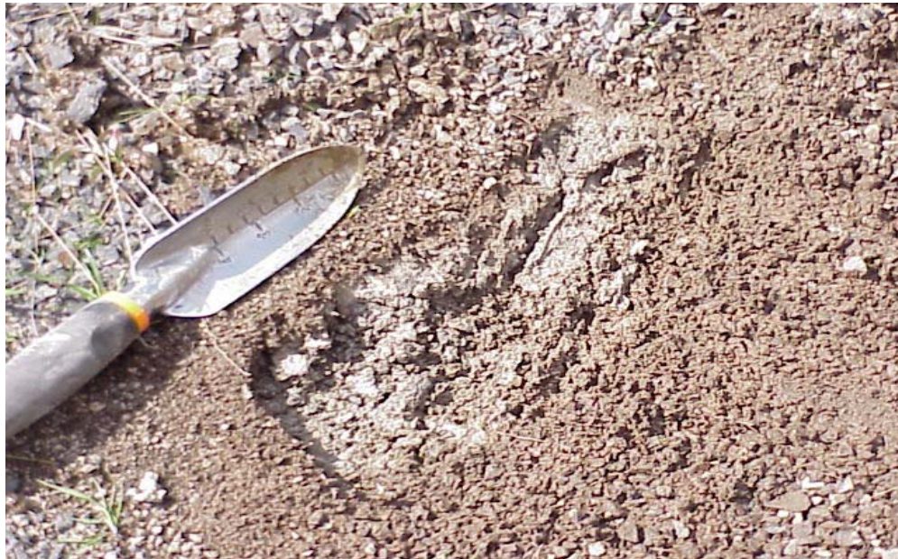
Figure 4.3 Presence of Slurry at a location on SR-195
