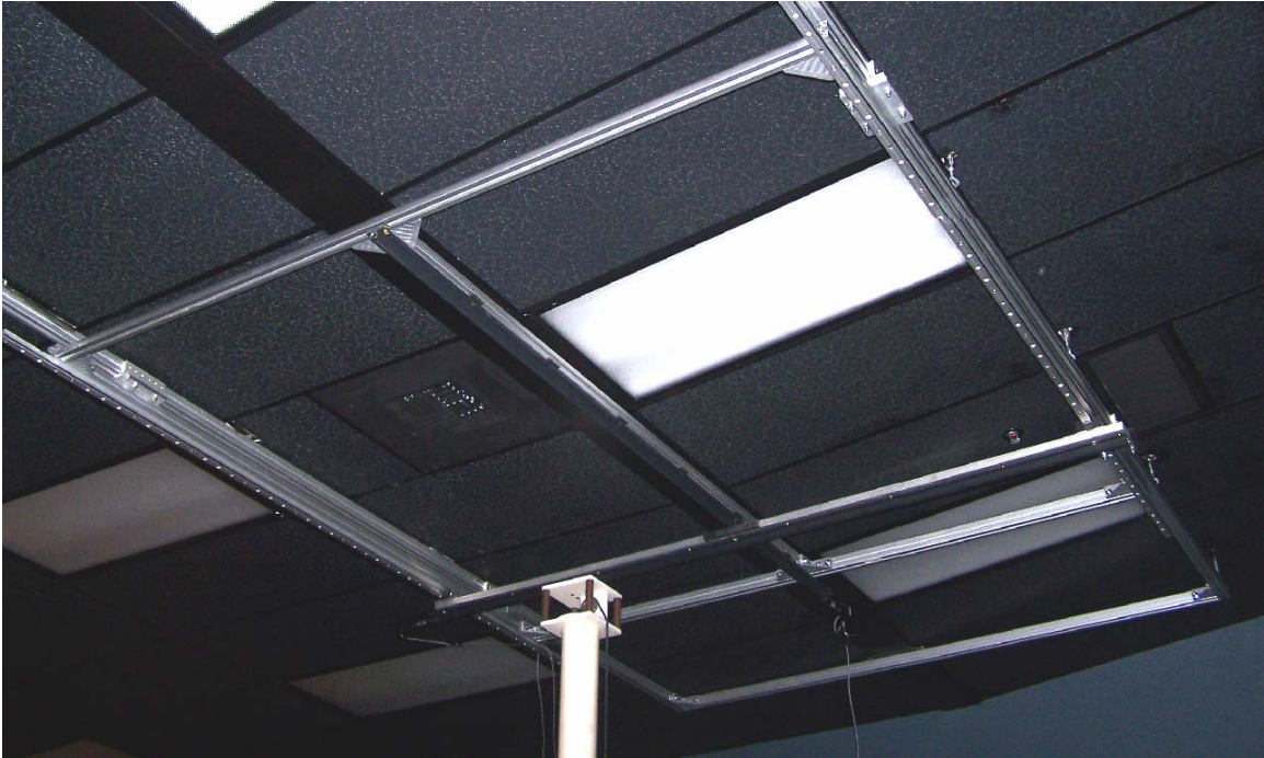
Figure 6.10: Calibration Device Installed
