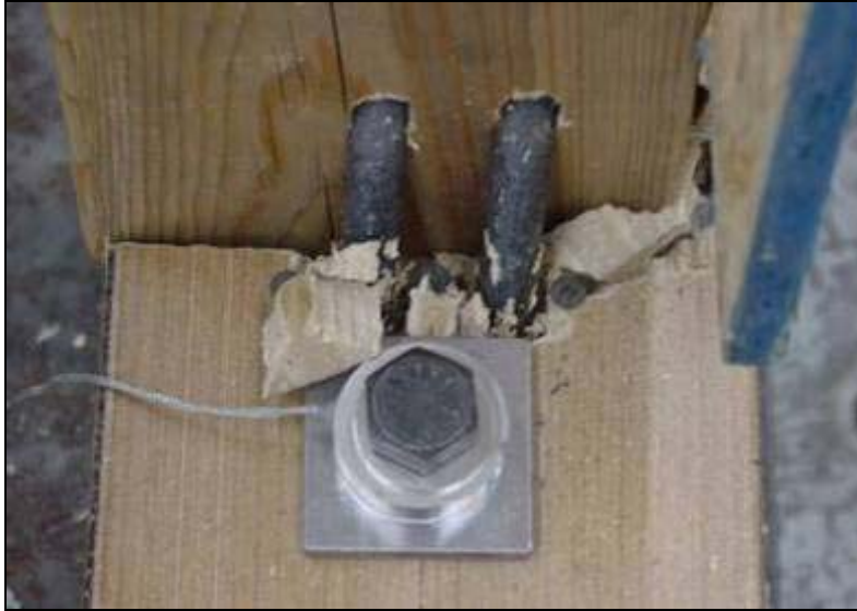
Figure B.5 End stud failed connection (top view): dowels yielded, top flange crushed, sill cracked through
