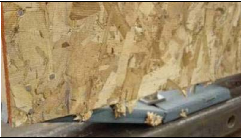
Figure 4.7 Nail bending and tear-out from sheathing and sill plate at loaded end of wall
